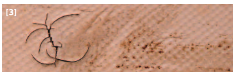
Illustrations: [1] Hailstones; [2] & [3] Damaged sealing membranes
